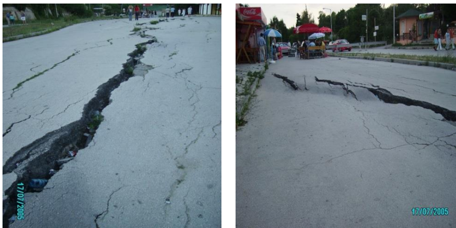
Figure 1: Cracks and subsidence in the area of Trifon Zarezan landslide.
