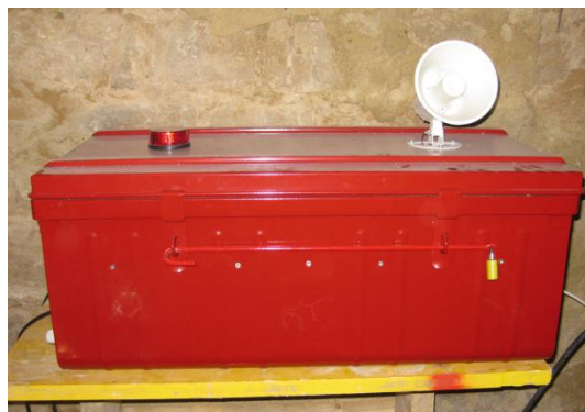
Illustration 8: Box for central computer and control system inclusive alarm system (optical and acoustical)
